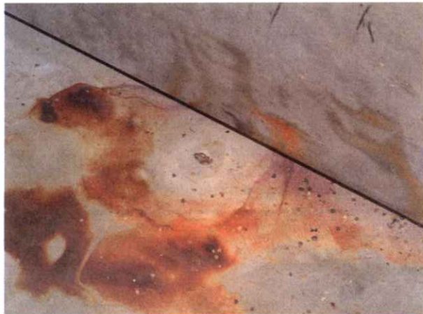
Pitting in a sand bed filter, caused by an aggressive biofilm [Microbiologically Induced Corrosion]. The brown ring (rust deposit) shows the rust hood that has been on top of the pit, in which very sour water caused the pitting corrosion. Picture: Jan Heselmans, Corrodium bv.
