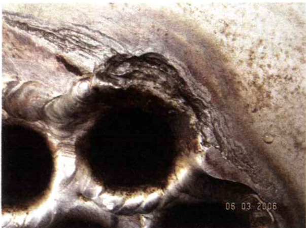
Crevice corrosion in duplex stainless steel seawater cooler. The corrosion can be stopped by use of pulsing sacrificial anodes. Picture: Jan Heselmans, Corrodium bv.
