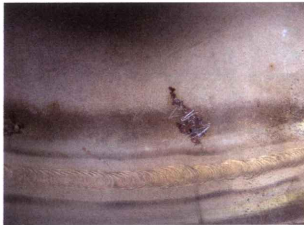
Inside of same pipe of picture A. After scratching rust scaling, pitting appeared to cause the leakage, which wetted the insulation material on the outside. The solution here is to change to duplex stainless steel as well because the PREN (pitting number) of duplex stainless steel is considerable better than the PREN of 304. For stress corrosion cracking resistance AISI 316 was no option. Picture: J. Heselmans, Corrodium bv.
