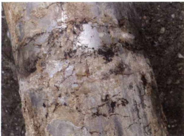
Stress corrosion cracking due to 'corrosion under insulation' from the outside to the inside of a hot water pipe. This is a AISI 304 pipe and the solution in this case is to change to duplex stainless steel. Duplex stainless steel is far less sensitive to chloride cracking than 304 and 316. Picture: J. Heselmans, Corrodium bv.
