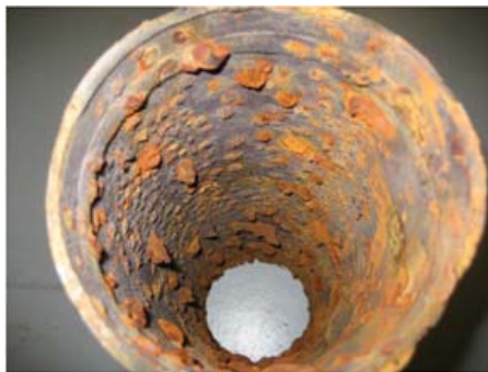
Figure 2. Steel 4" pipe affected by MIC (photo: MIC Europe private company)
