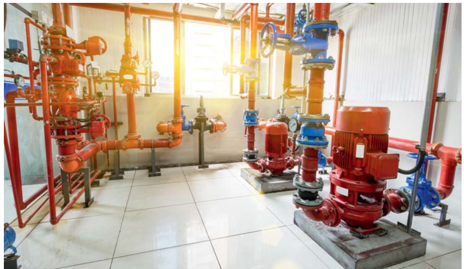
Microbiological induced corrosion is a serious threat to industrial fire protection systems and proper measures must be taken to detect and prevent it.
